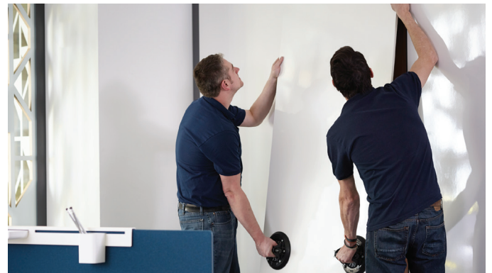
Step 4 – The Installing Dealer completes installation responsibilities to the customer’s satisfaction, on time and within budget.
